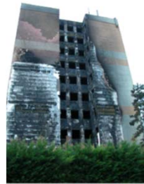
France 2010 EIFS façade Dumpster fire 7 fatalities
