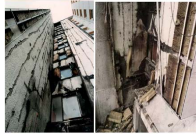
UK- 1991 Cavity wall façade Dumpster fire
