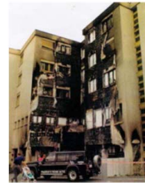
Munich 1996 EIFS façade Dumpster fire
